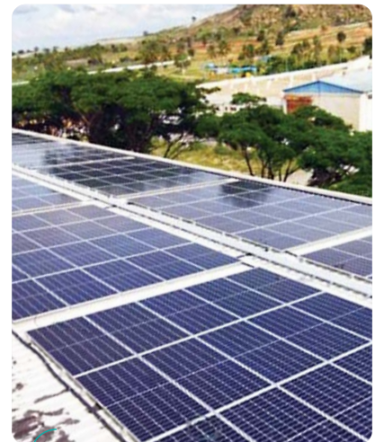
○ Expanding roof top solar application in EyeCare plant
