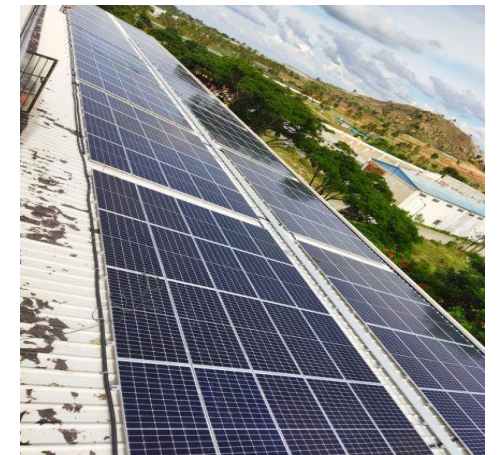
Roof top solar in Eyewear plant – Approx savings 5L units per year 56
