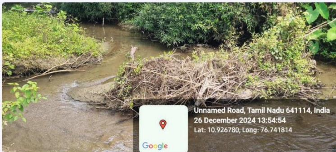
Severe silt formation and vegetation obstructing water flow — pre-intervention
