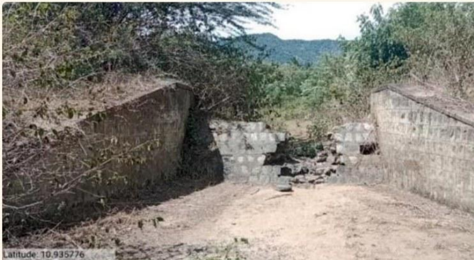
Check Dam #6 — only wing walls and severe damage to weir wall at baseline.
