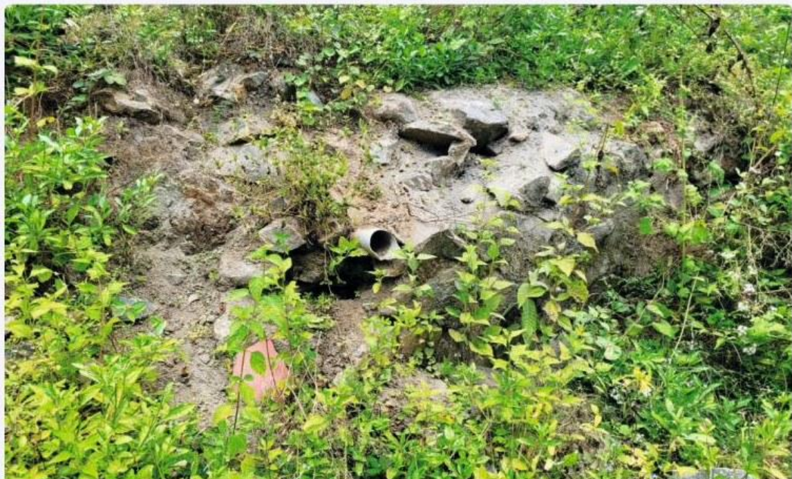
Outlet pipe from a nearby institutional campus discharging into the stream
