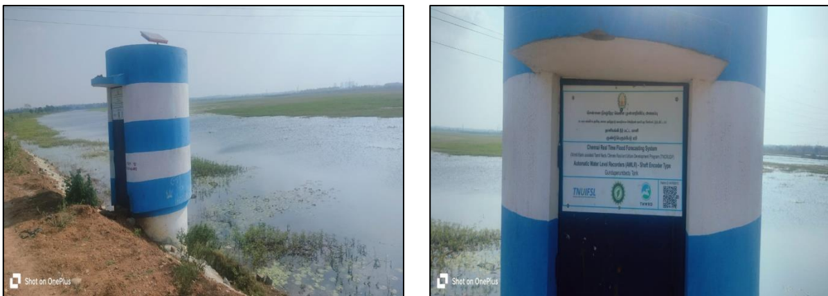
Figure 2.8: Automatic water level recorder installed at the lake
